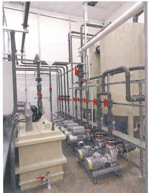
Pumps and tanks of a coolant processing system for the production of ophthalmic lenses
