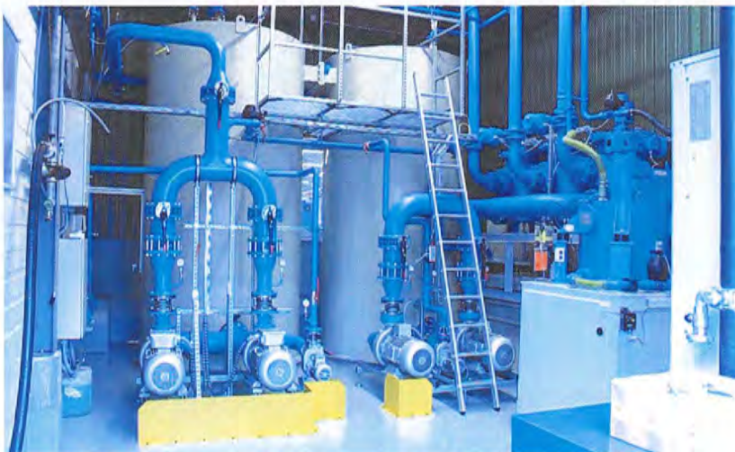
Centralized supply system for 25 grinding machines with back wash filters and centrifugal separators for secondary treatment
